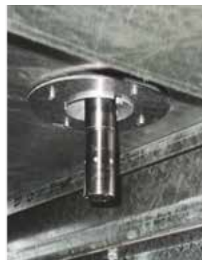
Typical sensor installation
