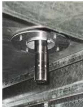
Typical sensor installation
